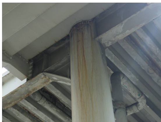
柱鋼管の塗膜劣化, 腐食
